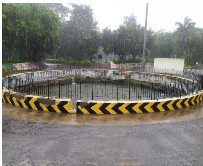
Rain water Harvesting Pond (4250m 3 )
