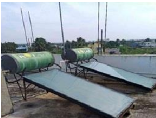
Solar Water Heater
