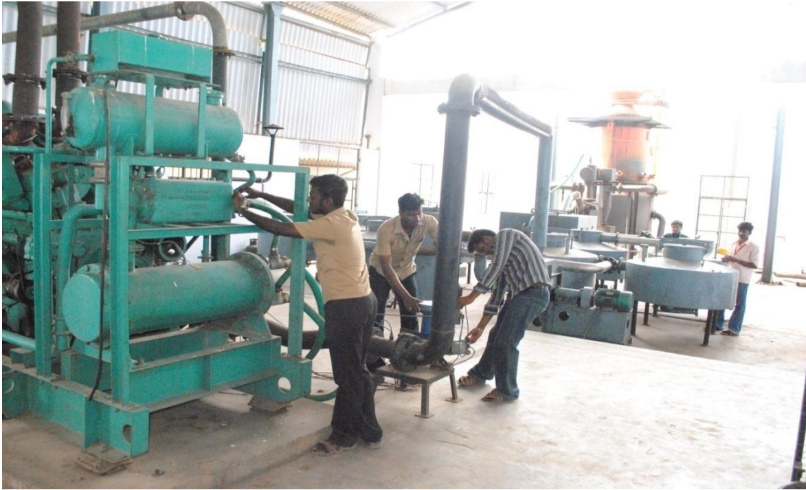
200 kWe bio mass gasifier for power generation (100% producer gas mode) Funded by MNRE, Govt. of India
