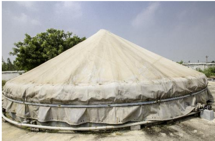
Anaerobic Digester of Biomethanisation plant
